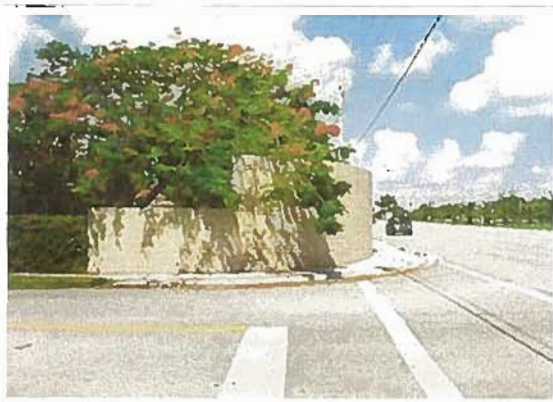
Figure 15. Barrier curved inward towards the community photo #2617
